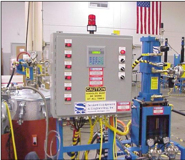
System control panel shows system HMI and temperature controllers for 6 heat zones (2 tanks, 2 hoses, meter A and B)
